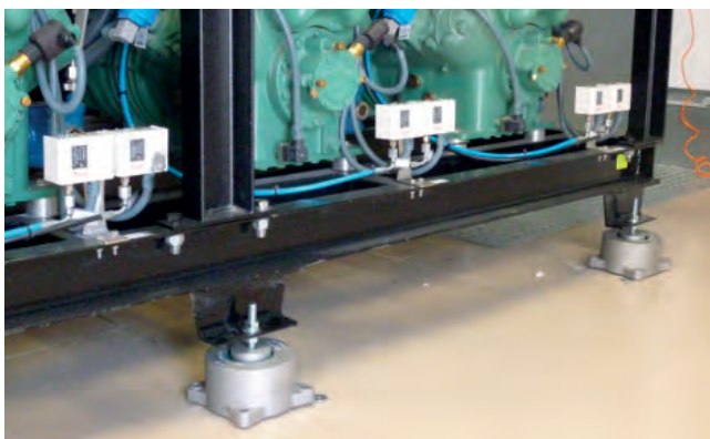
Example of installation on a HVAC equipment
