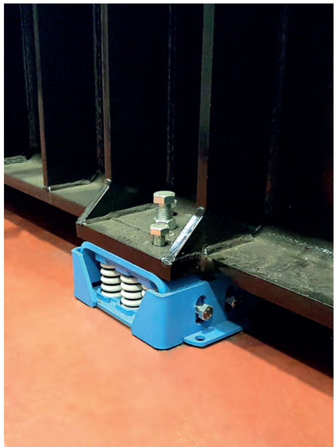
Generator set insulated with VIBRABSORBER+Sylomer®
